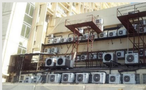
Figure 38: Split unit sprawl is a bad sight and often a waste of energy and money Source: GreenfieldCities
