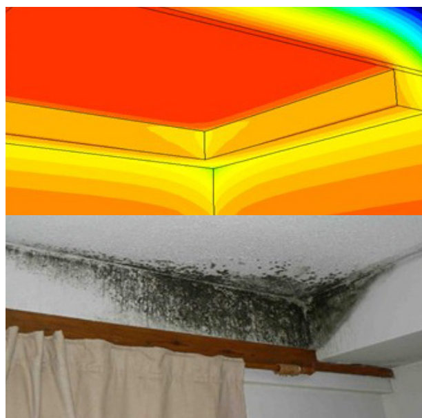
Figure 32: Thermal bridges may be the cause of mold problems
