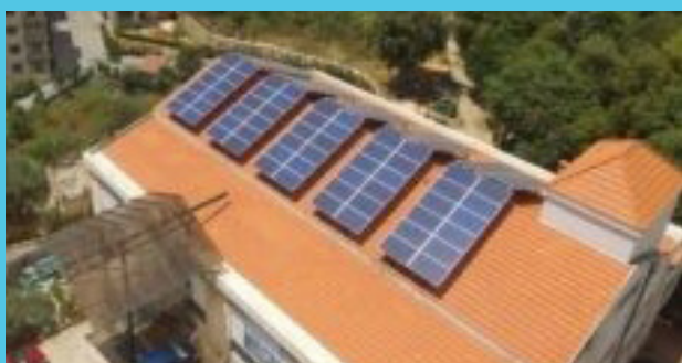
Figure 53: A hybrid on/off grid PV system in Baabdat Source: IBC Solar
