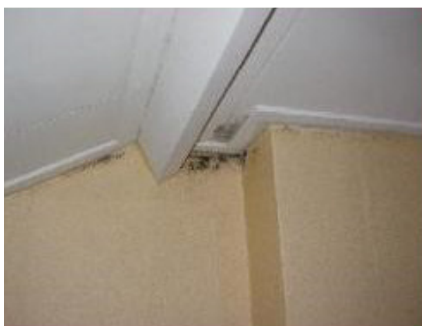
Figure 34: A thermal bridge causing mold near the connection to a balcony (below) is clearly visible in infrared imaging (above)
