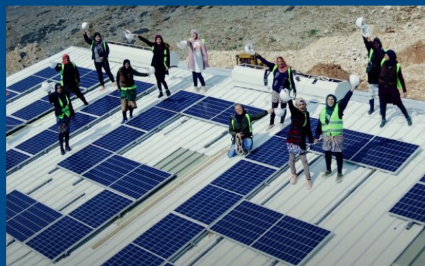
Figure 61: RiSE Solar project in Lebanon
