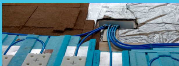
Figure 63: Example of a retrofit PCM assisted heating and cooling floor in an apartment
