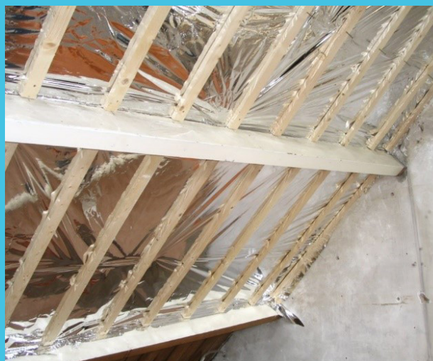
Figure 29: Insulation of a pitched roof can be done with foam or woolly materials, but also using several layers of heat reflecting foils, separated by air gaps. Recticel
