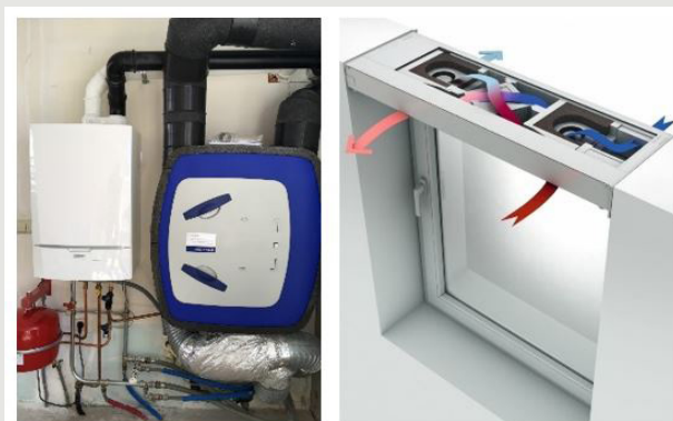
Figure 9: Heat recovery ventilation with over 90 per cent efficiency can be used in buildings of every size. The blue box on the left is a single home system Aqaba Residence Energy Efficiency
