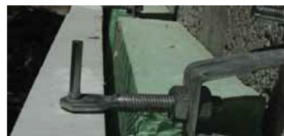
Figure 26: Extruded polystyrene insulation with wall renovation: new stone cladding in Dutch Embassy Amman- Source: Florentine Visser
