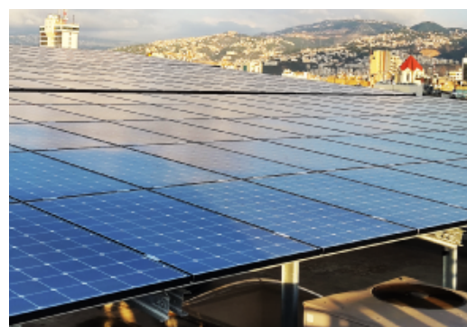
Figure 9. MEW Solar PV System
