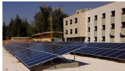
Figure 6. Ablah Medical Center Solar PV System
