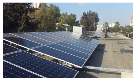
Figure 7. Qobbeh Medical Center Solar PV System
