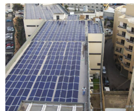
Figure 4. FDC Solar PV System
