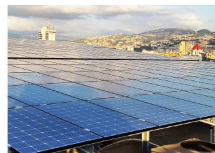
Figure 3. Libanjus. Solar PV System
