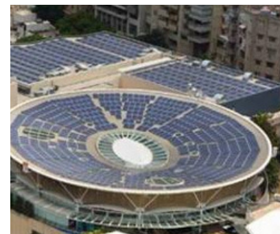
Figure 10. Parissis Steel Engineering Factory Solar PV System
