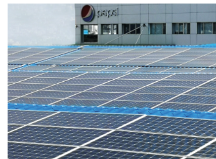
Figure 2. S.M.L.C Pepsico. Solar PV System
