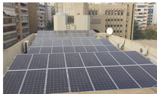
Figure 8. El Helou Barrack Solar PV System
